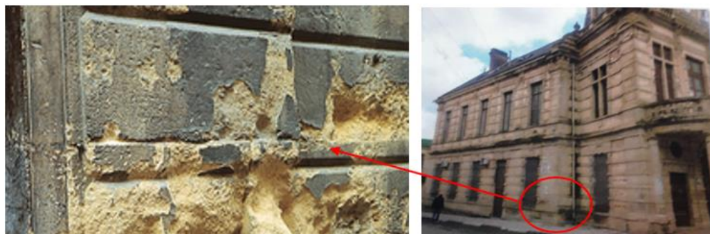
Fig. 4. Alveolization on the North Facade
