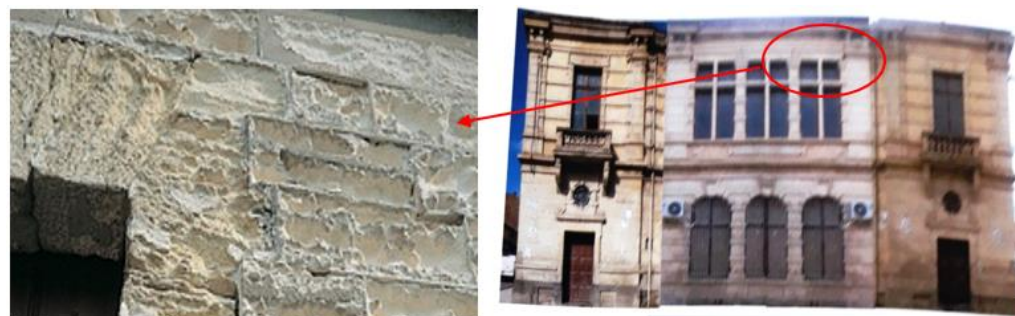
Fig. 5. Dissolution on the South East façade
