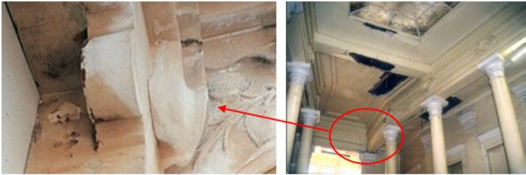
Fig. 6. Efflorescence on the Main Entrance
